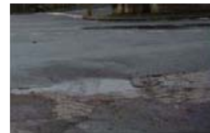
Photo 28. Visible stone sette in the highway at Occupation Road
