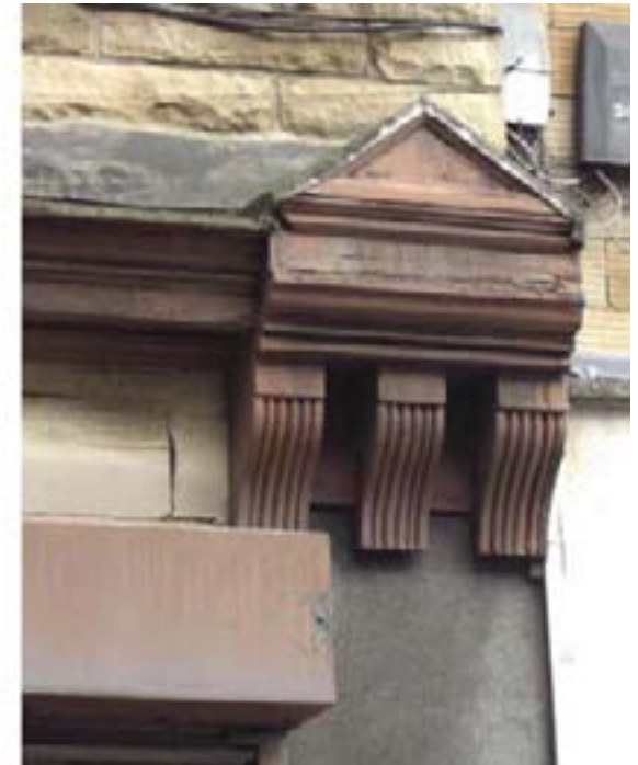
Victorian shop window detailing in a poor state of repair and covered by inappropriate materials and rolling shutter box.
