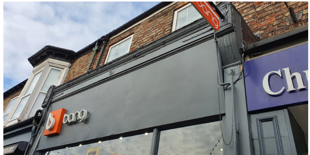
The blind box and fittings for an historic awning built into the cornice are clearly visible in this image above the overly-large fascia. Every effort should be made to preserve and reinstate such features
